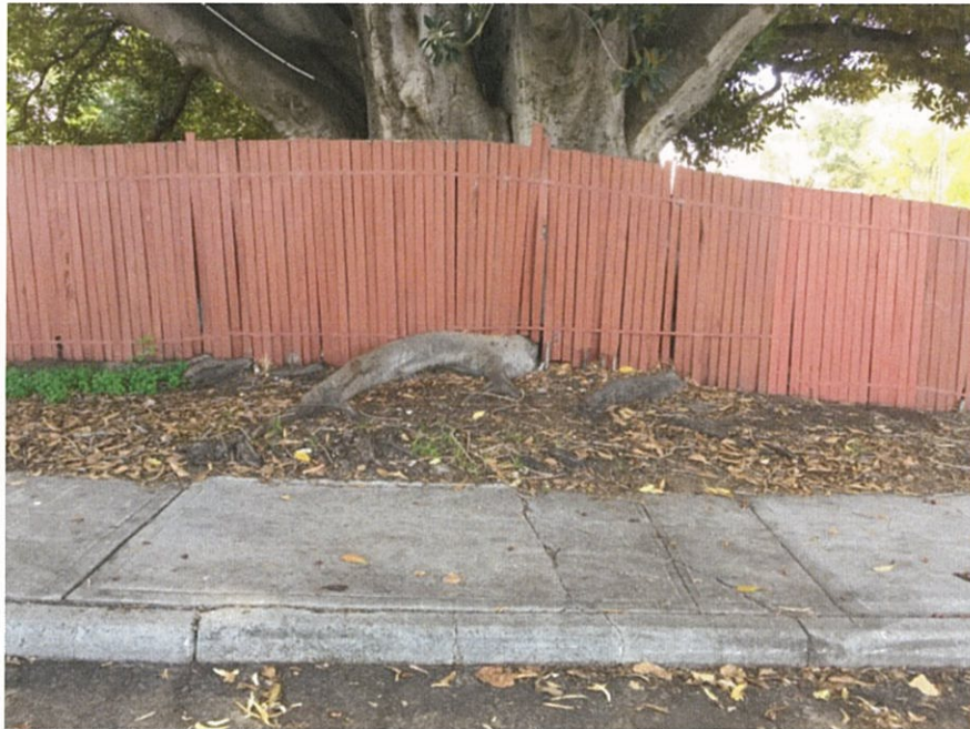
Figure 4. A minor root/ fence conflict was visible on the south side and is typical where a lightly-loaded structure such as the fence is located within the structural root zone of a large maturing tree, and any future fence repair or replacement should utilise a pier and beam construction technique that spans the structure over the root plate of the tree; looking towards the north.
